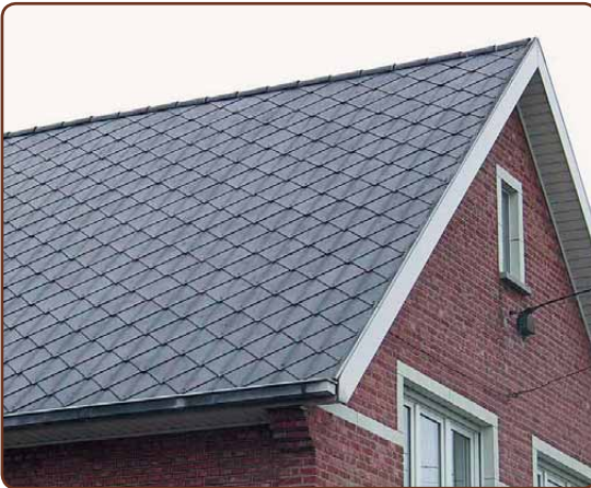
Dakleien in asbestcement
